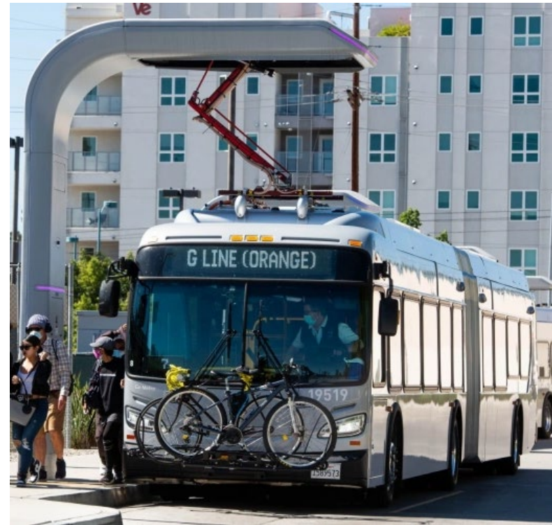
North Hollywood On-Route Inverted Pantograph Charger
